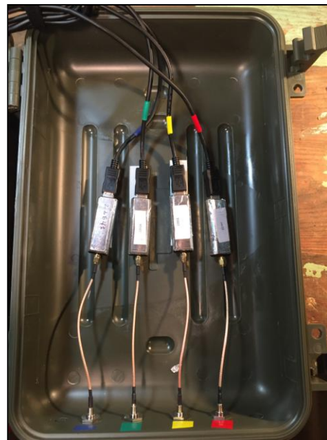
Figure 10: A color coding scheme for your antennas is helpful when troubleshooting a tower. Colored tape is also used outside the SG on coaxial cables and antennas, for easy reference throughout your system.
